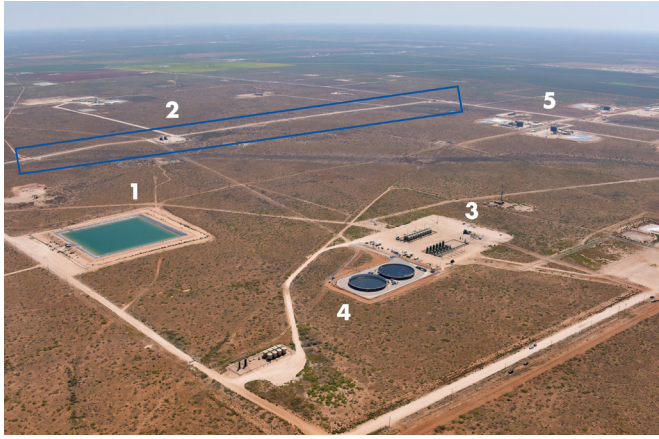
Figure 1. Water management infrastructure. This representative layout includes (1) fresh water storage, (2) a produced water trunk line system, (3) gathering and treatment facilities for produced water, and (4) produced water storage and blending tanks. The entire arrangement is strategically located in proximity to several active fracking locations (5).
