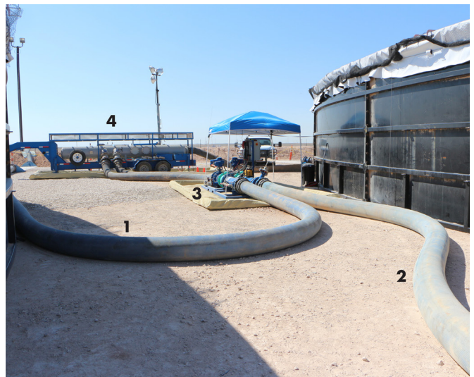
Figure 4. Automated blending components. (1) Fresh water inlet; (2) Produced water inlet; (3) Automated blending controller; and (4) Blending manifold.
