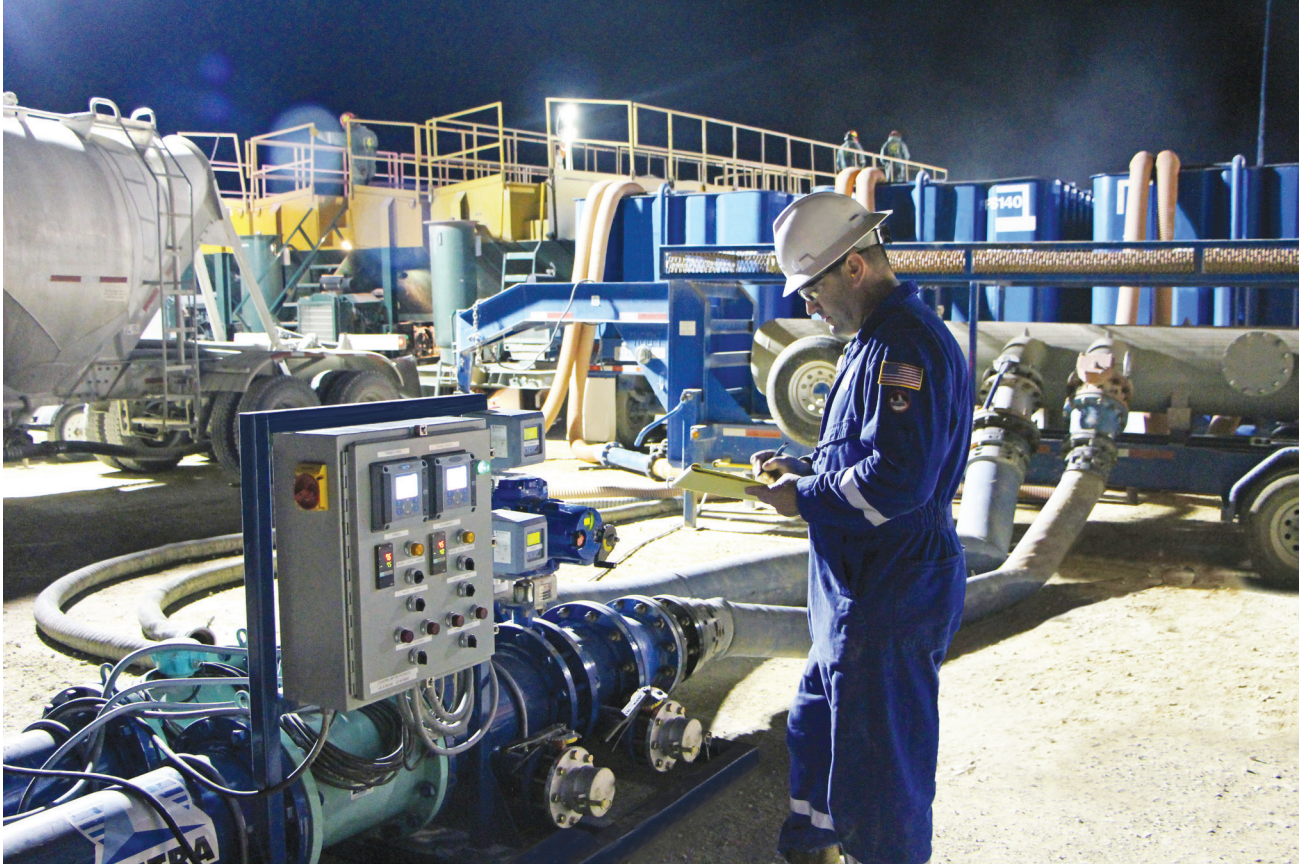
The frac water blending system includes an automated blending controller, coupled with an on-the-fly blending manifold. The combination provides accurate parameter-based blending and consistent blend quality, whether directly filling frac tanks or transferring to another location. (Source: TETRA Technologies)
